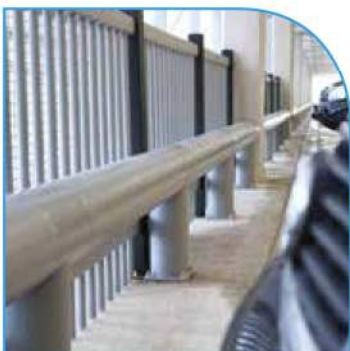
Car Park Barrier with Anti-Climb
